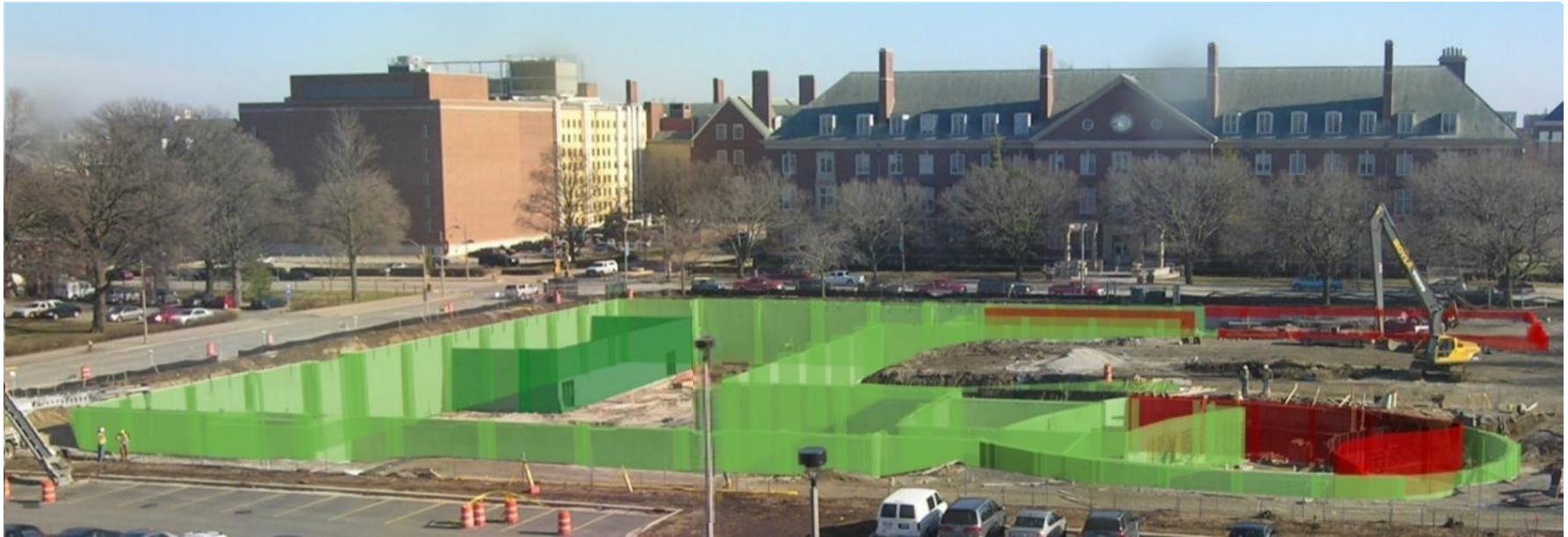
Project: College of Business Instructional Facility, Photograph Courtesy of Facilities & Services, UIUC.
